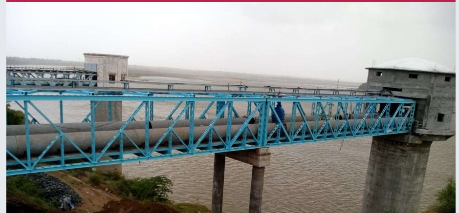
Intake Well 25 MGD at Narmada River Nand
